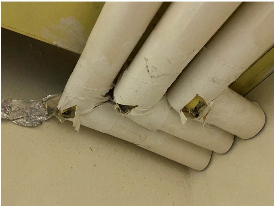
Confirmed Asbestos, S0011A-C, Piping, Heating Water Supply, Aircell, Maintenance Office (Location #: 7)
