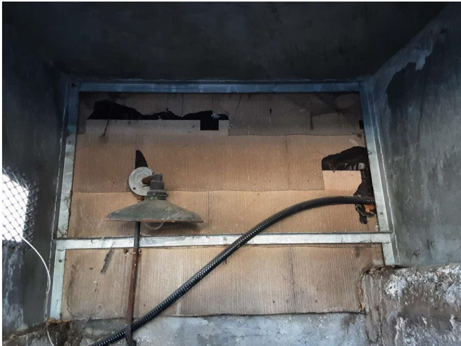
Confirmed Asbestos, S0021A-C, Wall, Cement Product (Transite siding), Boiler Room And Stairwell (Location #: 24)
