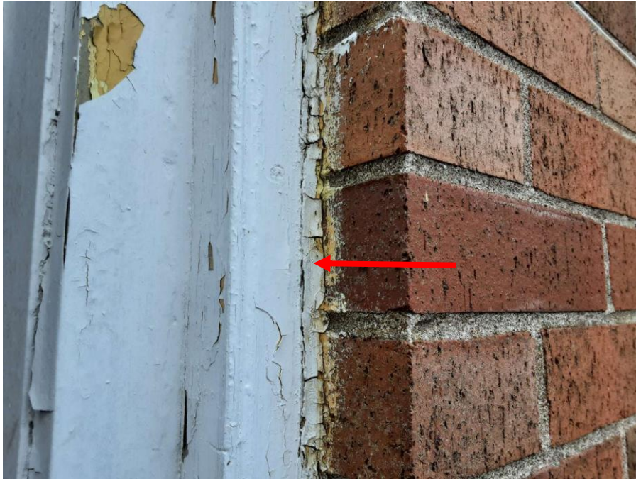
Confirmed Asbestos, S0002A-C, Wall, White Caulking, Exterior (Location #: 1)
