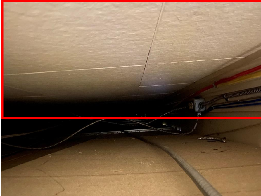
Presumed Asbestos (V9500), Glue-on ceiling tiles above lay-in ceiling tiles, Hallway (Location #: 11)
