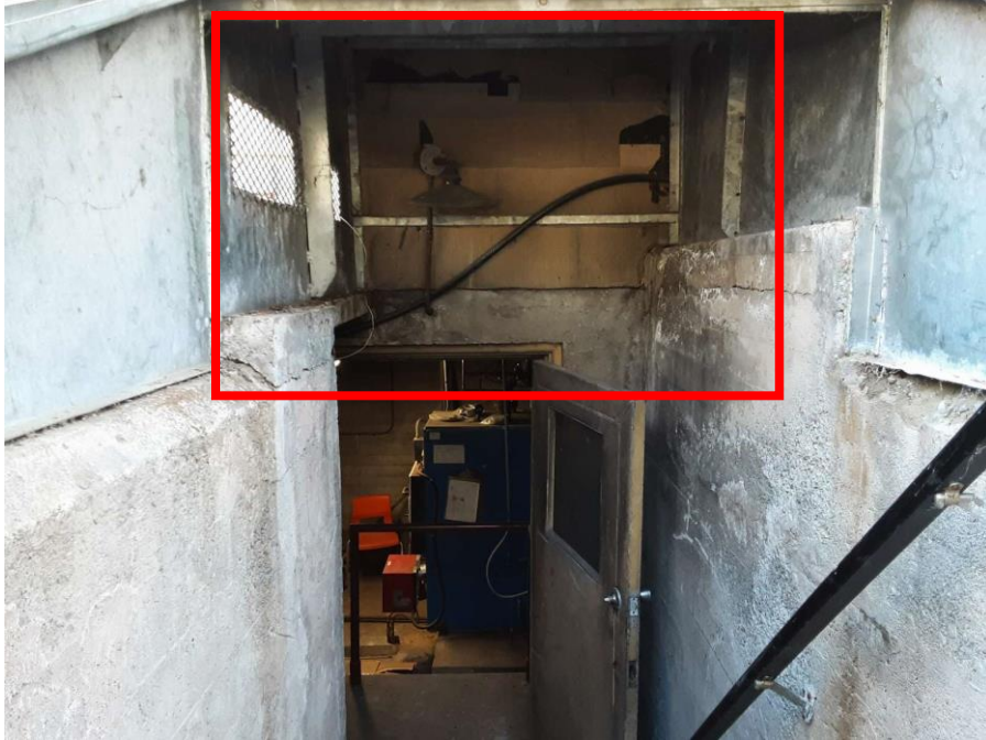
Confirmed Asbestos, S0021A-C, Wall, Cement Product (Transite siding), Boiler Room And Stairwell (Location #: 24)
