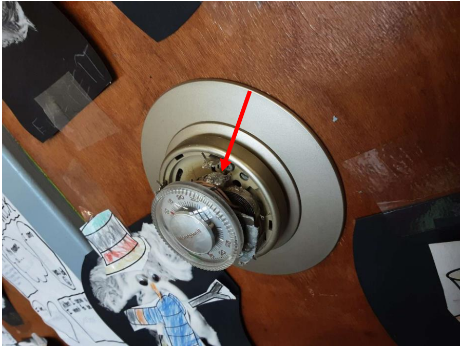
Confirmed Mercury , Liquid mercury in thermostat ampule, Classroom 6 (Location #: 2)
