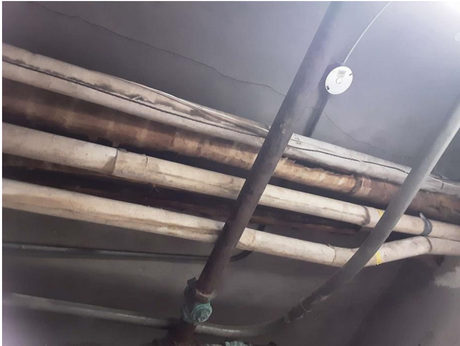
Confirmed Asbestos, S0011A-C, Piping, Heating Water Supply, Aircell, Oil Tank Room (Location #: 25)
