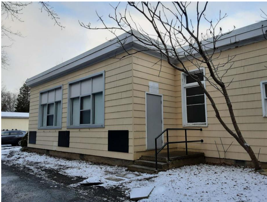
L0001, Yellow paint on wood siding, Exterior (Location #: 1)
