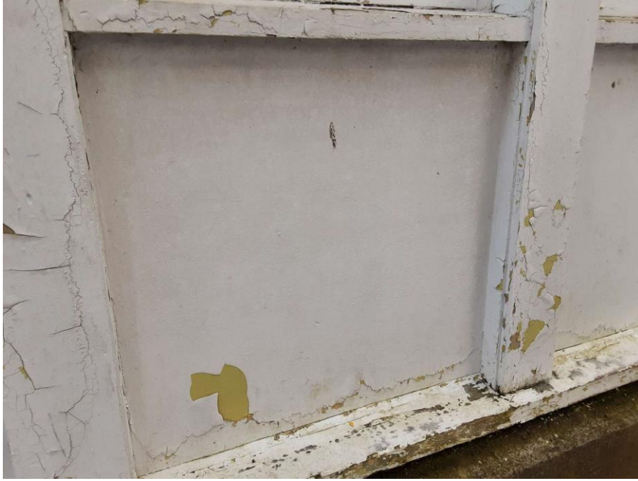
Confirmed Asbestos, S0001A-C, Wall, Cement Product (Transite panels), Exterior (Location #: 1)
